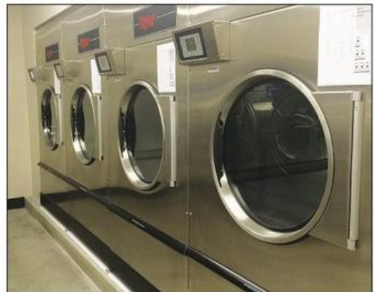
With the new washer-extractors and the pictured dryers, WSU equipment staff can turn around daily football laundry in just over an hour.
