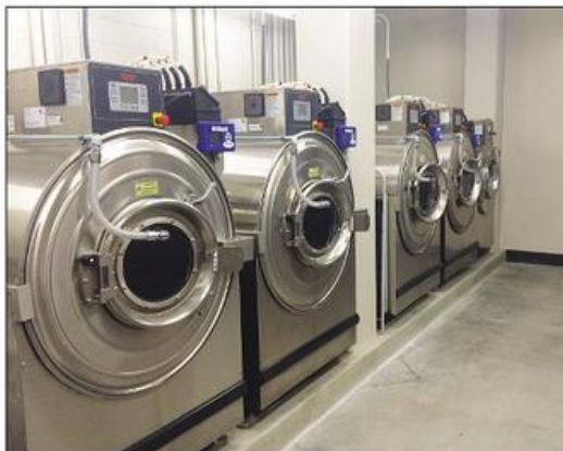
Washington State's washer-extractors are only 10 feet away from the chutes where the soiled laundry is deposited.
